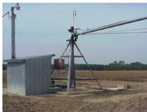
Figure 2. A pivot point or "pad" and pump house
